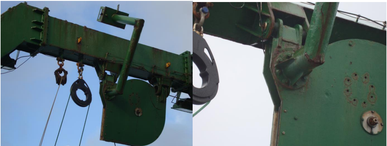
Pictures of the A-frame flag block counter weight on the R/V Kilo Moana on December 12 th , 2018.
